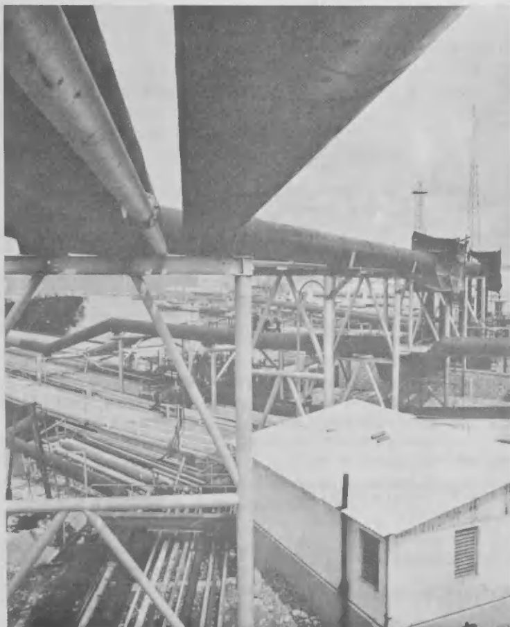
Partial view of 36-inch line (at extreme right) running zigzag over high trestles over pipe banks near Finger Pier No. 3.
